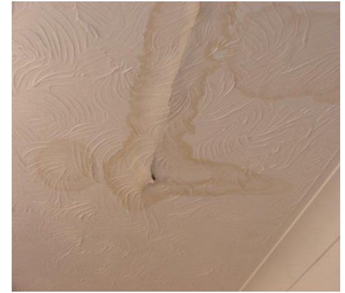
Damage after bath seal failed
